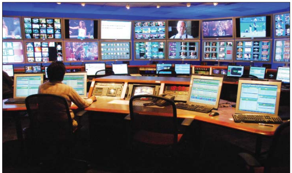
The Broadcast Facilities operations center
